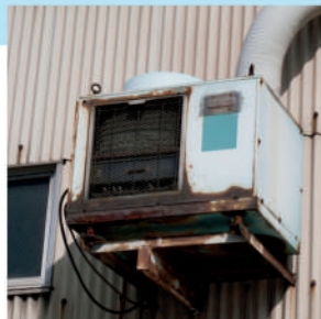
Large heat exhaust systems
